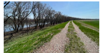
Inaccessible Levee Path
